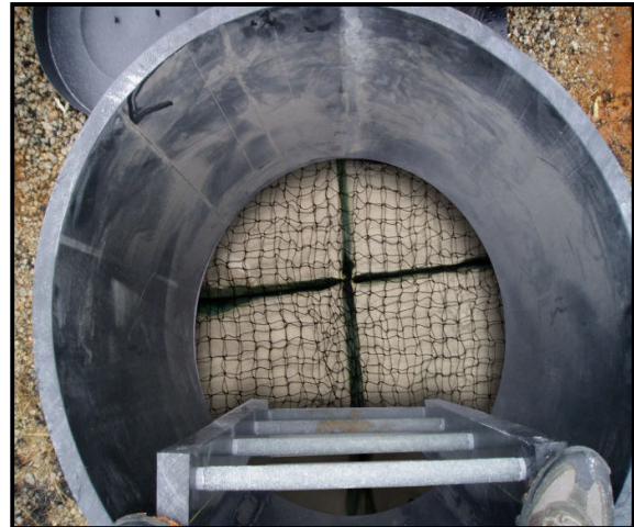
Ingress/Egress ladder and filter containers covered by cargo netting.
