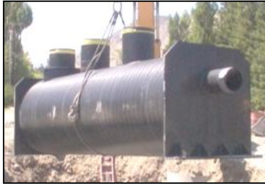
Filtration chamber of Aqua-Filter™ system being lowered into place. Access risers are visible along the top length of the chamber.
